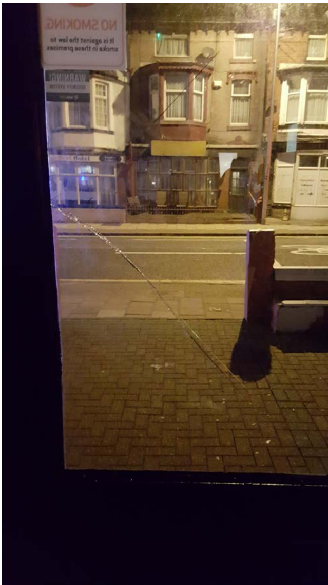
Large crack in the glass to the main front, further evidence of disrepair.
